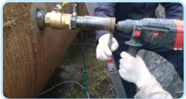
Insertion Transducer Installation
