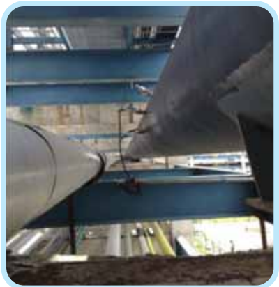
Power Plant Circulation Water
