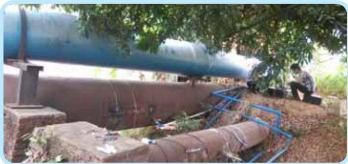
DN800 Water Supply
